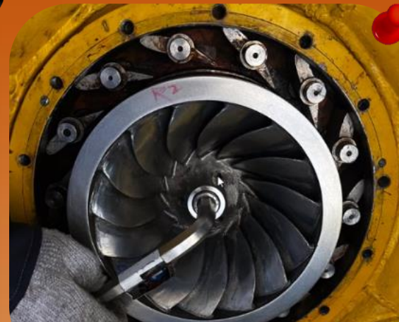
Installation of the Francis runner designed by TTL for Nakayama Iron Works Pvt. Ltd. Japan
