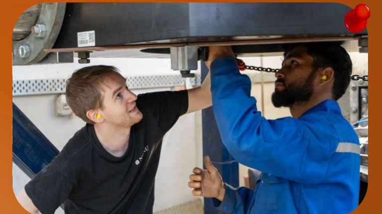
Assemble/Disassemble works of the Francis turbine at TTL in the presence of the technicians from the Waterpower Lab, NTNU
