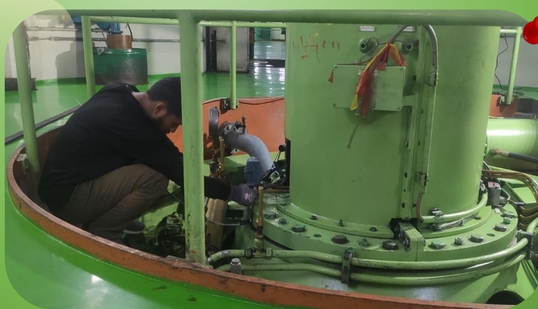
Visit to Marsyangdi HPP by Mr. Prajwal Sapkota and Mr. Bhuwan Bhatara in the course of CMHydro and RenewHydro projects running at TTL
